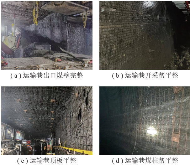
图 17 2201 工作面停采期间煤壁及运输巷道围岩情况 Fig. 17 The conditions of the coal wall and the surrounding rocks of the transportation roadway during the shutdown period of 2201 working face
