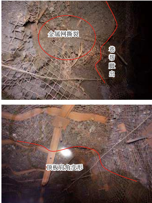
图2 现场破坏情况 Fig. 2 The filed destruction situation
